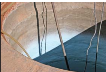
The bright, highly reflective blue epoxy coating nears the top of a manhole.
