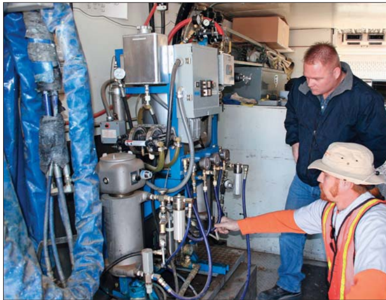
Don McDowell looks on as operations manager Tom Van Duinen checks the pumping system. This is where the epoxy components get their final heating and pressurization.
