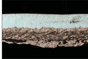
This close-up shows a section of bad concrete that broke from the side of a manhole. Note the epoxy's surface penetration and solid adhesion.
